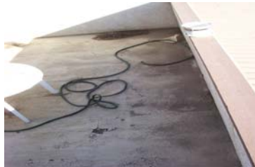
Lack of maintenance has allowed UV to destroy this expensive coating!
