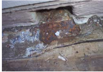
Rusted metal is revealed after old coating was removed. This scupper must be replaced to properly waterproof the deck.
