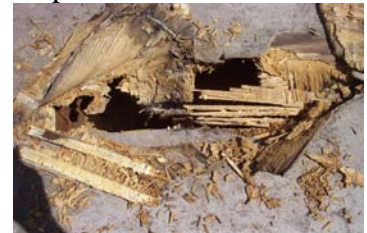
Dry-rotted substrate needs to be replaced before new decking can be installed.
