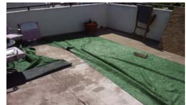
Indoor/outdoor carpeting is bad for decks, they trap water underneath!
