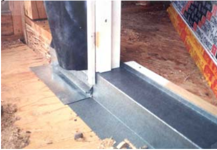
This is an example of a sheet metal door pan. Code requires all terminations and doors be flashed properly.
